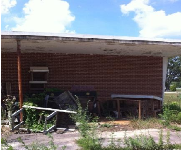
The abandoned warehouse.
